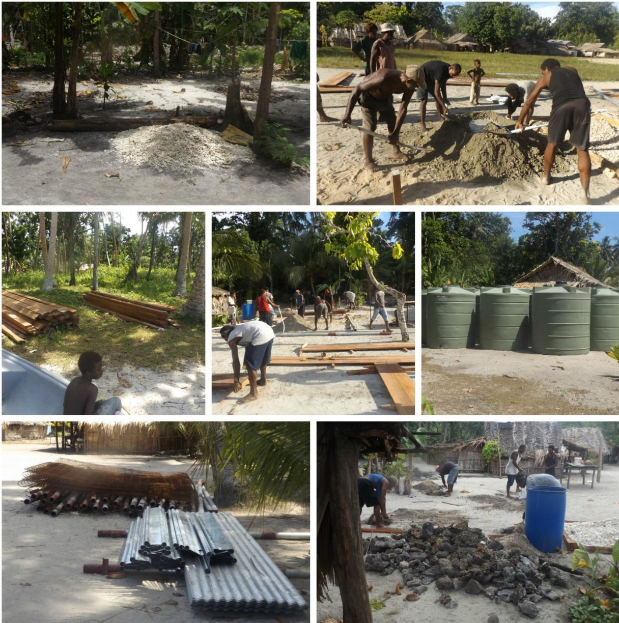
Subi Construction and Santa Catalina community members working together to get the rainwater harvesting system constructed and installed.
